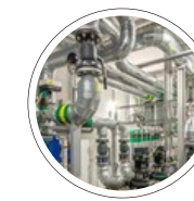
Fan and Water pump
